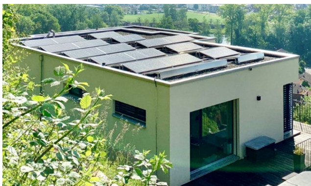
© Helion Energy AG
