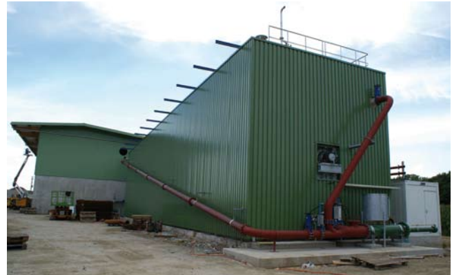
Digester. Source: Eric De Lainsecq (Domotech)
