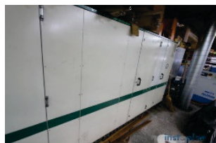
Figure 8 : Ventilation production monobloc extraction
