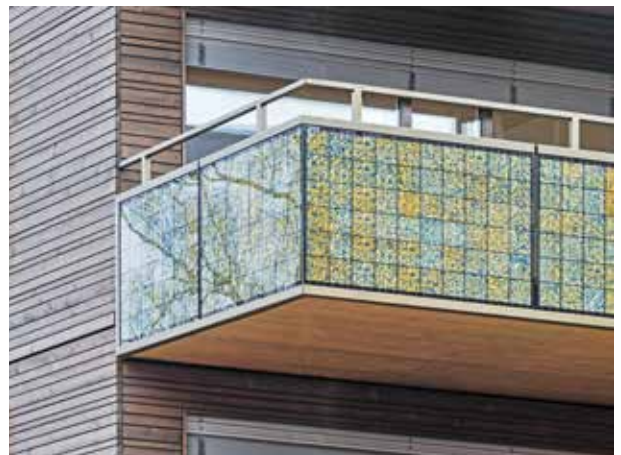
BALCONY BALUSTRADES WITH POLYCRYSTALLINE PV-MODULES FOR A MULTI-FAMILY HOUSE ON ZWYSSIGSTRASSE, ZURICH
