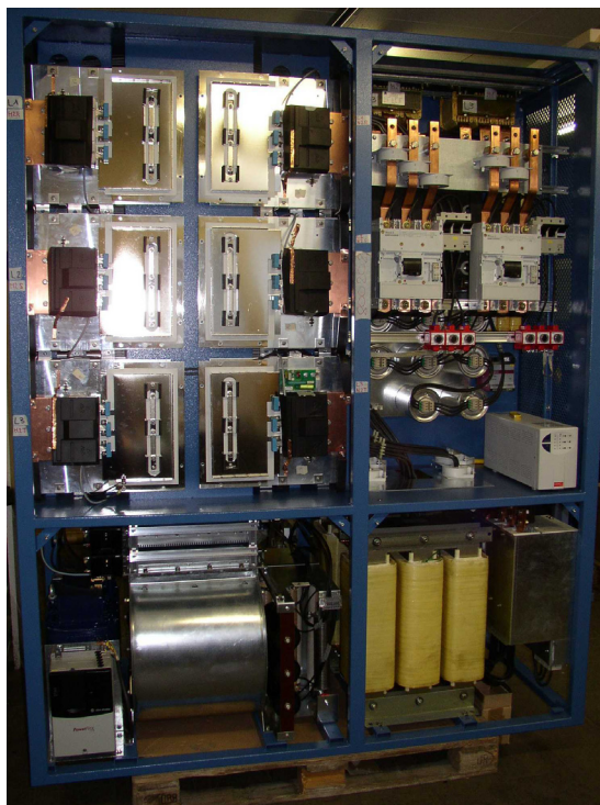
Figure 3: Prototype of a 1,200 kilowatt converter shortly before completion (source: Technocon AG)
