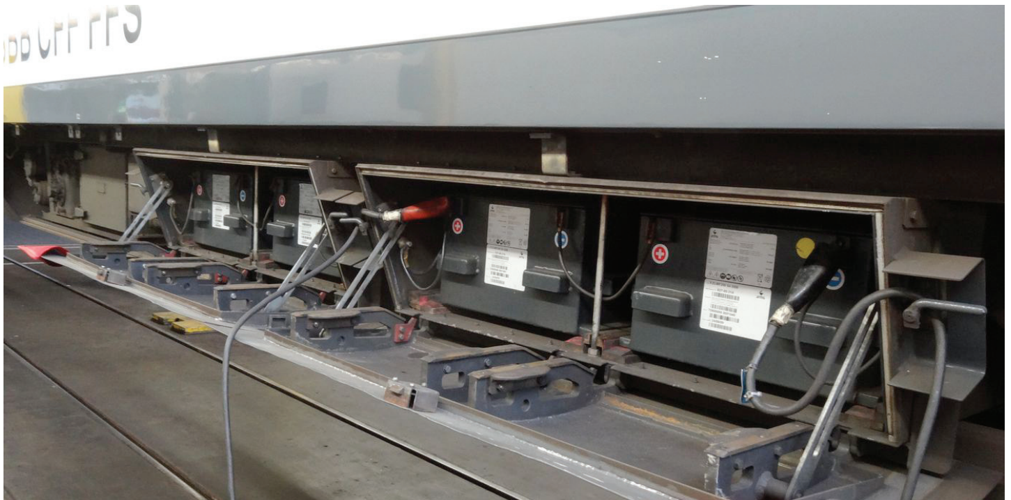
The EW4 travel wagon carries two parallel 36 V battery compartments, each currently housing in four hutches an 18 V lead battery. Photo: SBB
