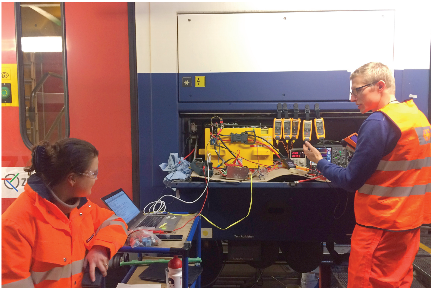
Lea Steurs from the SBB (management and logging of the test procedure) and Christian Vögtli from the BFH test the prototype battery on the regional train wagon DPZ. Photo: SBB
