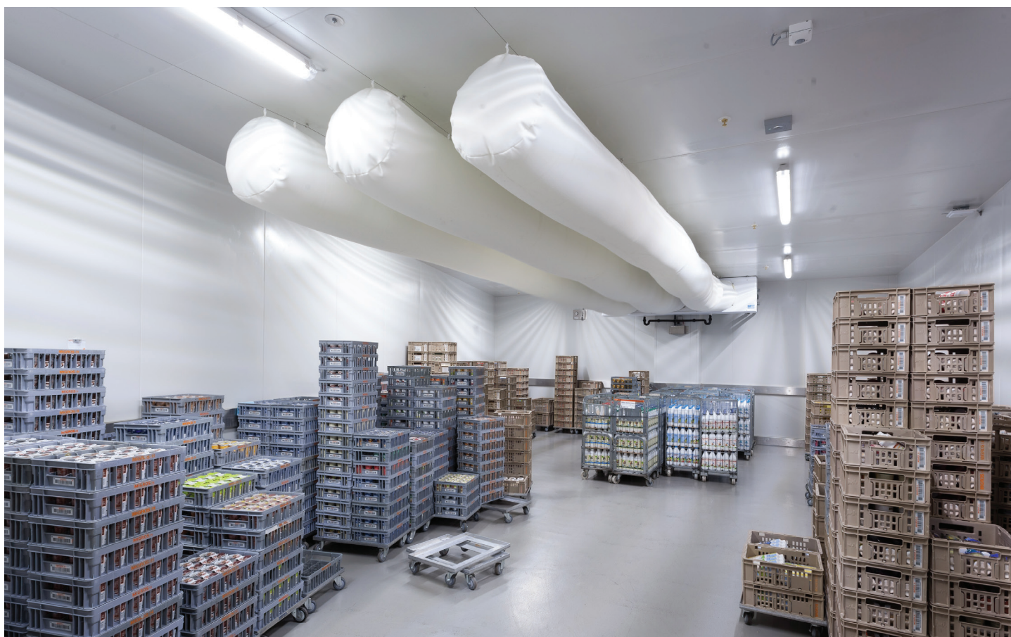
A cooling room of the Migros branch in Ibach (Canton Schwyz). The three textile tubes on the ceiling provide the room with + 1 ° C air. Photo: Frigo-Consulting
