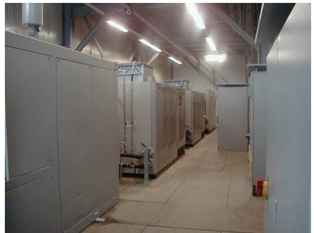
Fig. 2: Compressed air system
