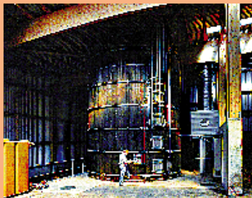
A composting and fermentation plant at Baar processes 18'000 t of bio-waste each year. This new process is even able to supply surplus electricity and is also free of waste water thanks to a bio-filter (photo) for cleaning exhaust air.
