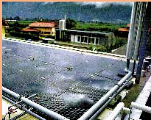
New type of solar roof made of integrated stainless steel absorbers without glass cover: 1/3 less yield than covered collectors but only a fraction of the cost. Photo: a test installation in Saillon.
