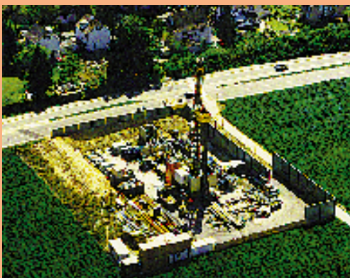
At the geothermal deep-drilling plant in Reinach, canton of Baselland, noise barriers were used to shield nearby residents from drilling noise. After the drillings were completed, the terrain was returned to its original state.
