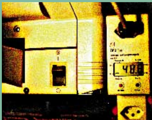
Switched off, but still drawing nearly 50W while on stand-by. »Secret power guzzlers« such as this photocopier were identified in Federal Office of Energy programmes, and manufacturers responded by making improvements.
