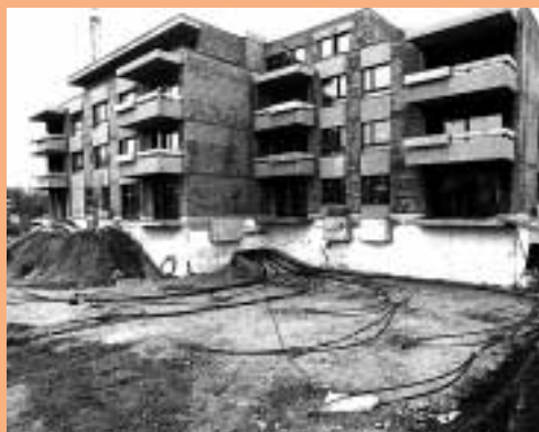
A dozen GP for heating an apartment block have already been sunk into the drilled holes. The pipes to the heat pump in the basement are still exposed before being covered with earth.
