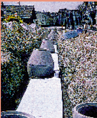
Waste heat storage for apartments at Buchrain with nineteen 200 mm geothermal probes (2 per shaft, 3 horizontal heat-insulated collection pipes).
