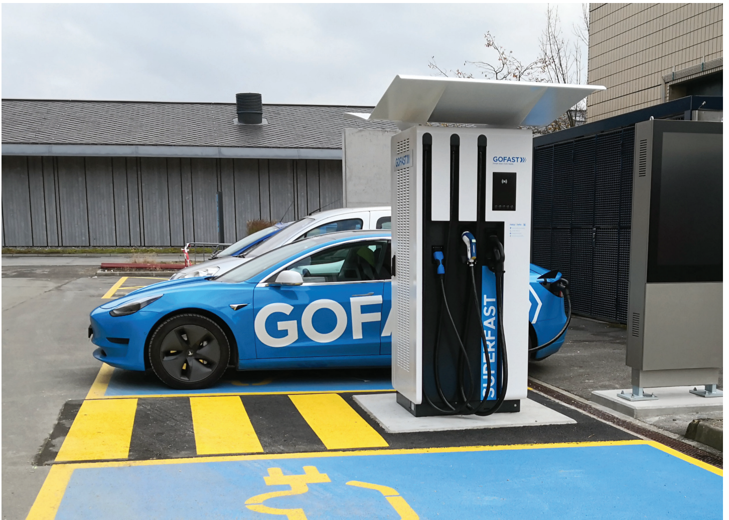
Charging station for two electric cars on the EPFL campus. Photo: MESH4U
