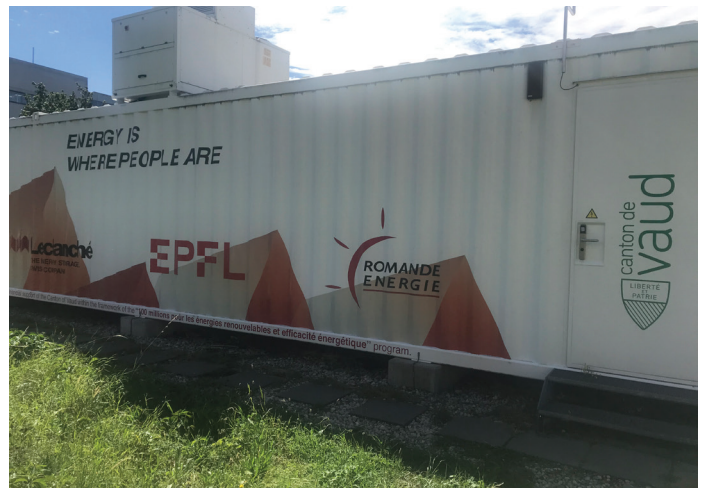
This battery storage system with a capacity of 560 kWh helped to operate the EPFL charging stations in a grid-friendly manner. Photo: MESH4U
