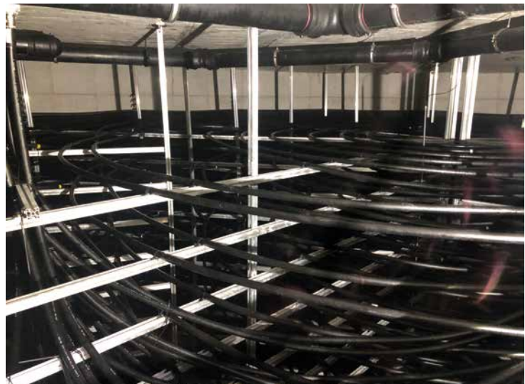
View of the inside of an ice storage tank before it was filled with water. Heat is extracted from the water during operation via the pipes arranged in a ring, which eventually causes it to start freezing from the bottom up. A free space was deliberately left on the very outside so that no ice would form there that could cause damage to the wall. The ice storage is defrosted by a second pipe system installed on the walls. The ice store therefore defrosts from the outside to the inside (source: Viessmann Schweiz AG).
