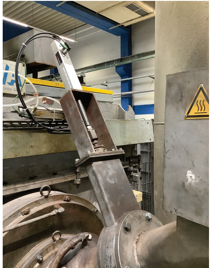
Stihl Kettenwerk is one of the companies that replaced compressed air cylinders with electric cylinders. Electric cylinders are likely to be superior to compressed air cylinders in terms of service life because of their high-quality components. Photo: Cyltronic
