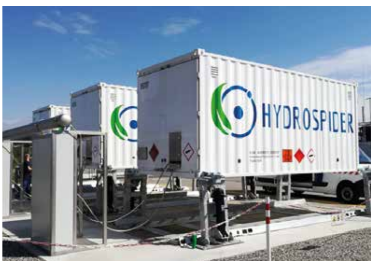
A 2MW electrolyser plant at the run-of-river power plant "Gösgen" will go into operation in 2020 to produce "green hydrogen" for fuel cell trucks. The picture shows tank containers, where the hydrogen produced is temporarily stored and which are used to supply the filling stations in Switzerland with hydrogen (Source: HydrosSpider).
