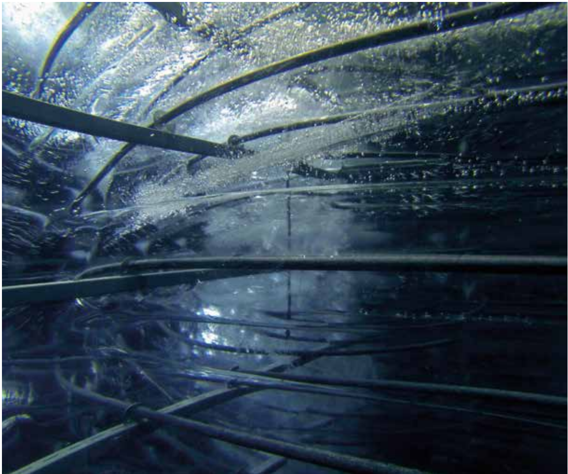
Underground ice storage system with a heat sink capacity of 30,000 kWh. Ice storage systems are latent heat storage systems with water as the storage medium, where the latent heat is used as storage during the phase transition from ice to water and vice versa. In the temperature range above 0 °C, they can also serve as sensitive heat stores (source: SCHNEPF Planungsgruppe Energietechnik, Nagold, Germany).
