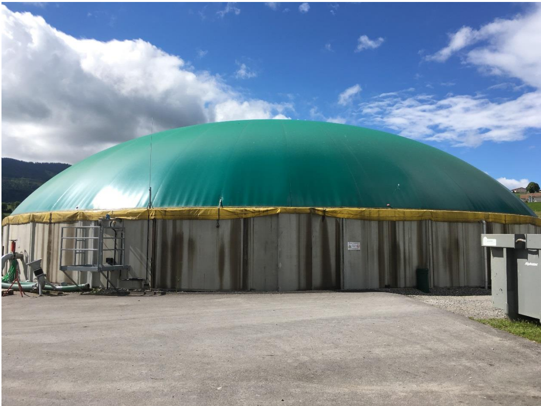
Biogasanlage in Mouret
