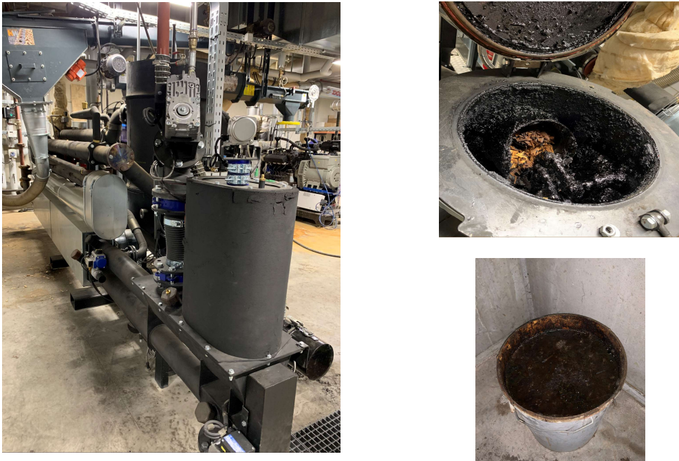
Figure 4.10: Gasifier CHP plant from Spanner Re 2 in Switzerland. Left: Gasifier. Right top: View into gasification reactor after operation. Right bottom: Liquid residues (tar). Photos: T. Nussbaumer, 2024.
