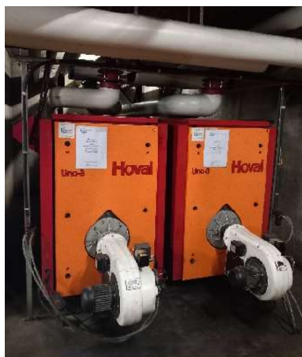
Figure 2 : Chaudières mazout – 2x 280 kW
