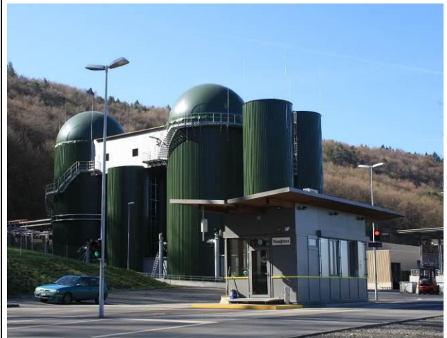
Biogasanlage KBA Hard, Beringen (SH)
